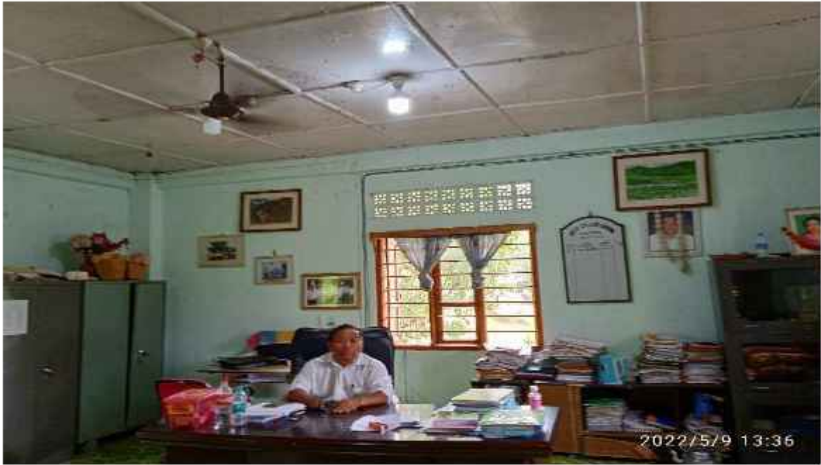
Pic 4: Use of Led bulbs in the Office of The Principal, Dr BD Thumdal
